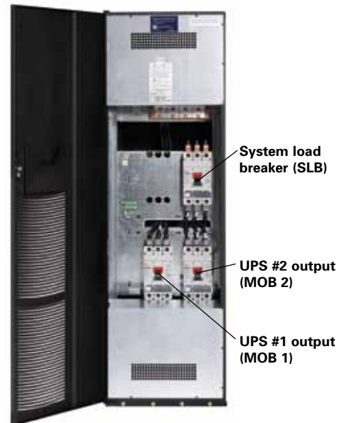
IAC-T Parallel Tie Cabinet
